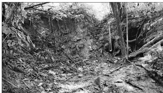
Figure 7. The upper part of one of a branch in gully system in Pogródka valley – effects of piping, developing along roots [in the background of the picture] [Photo by A. Solarska]
